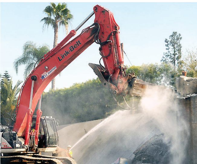
Crews demolish the existing abutments at the Colorado Boulevard bridge in Arcadia. Photo courtesy of Walt Mancini/Pasadena Star-News.
